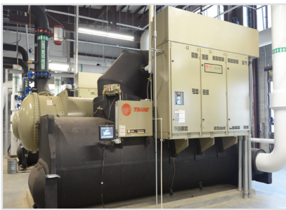
Comprehensive Maintenance Plans
